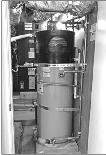
This small utility closet contains both the Griffiths' electric heat pump water heater (foreground) and their electric heat pump furnace's air handler (background).
