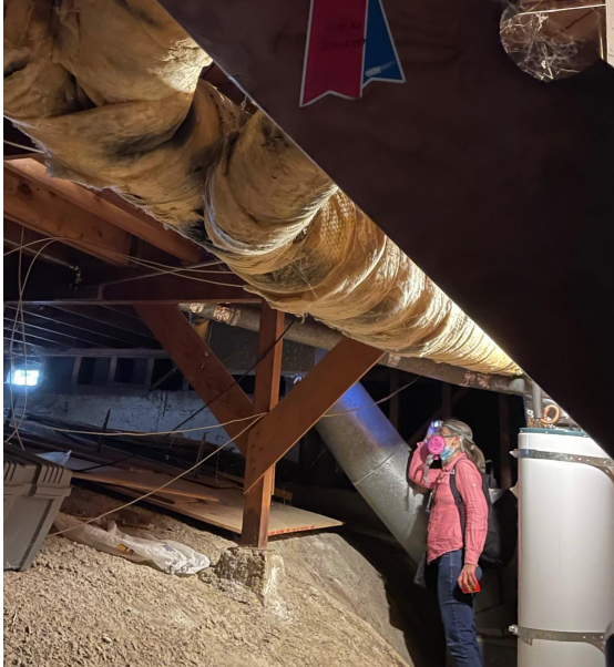
Today: 40-gallon gas tank WH in basement
