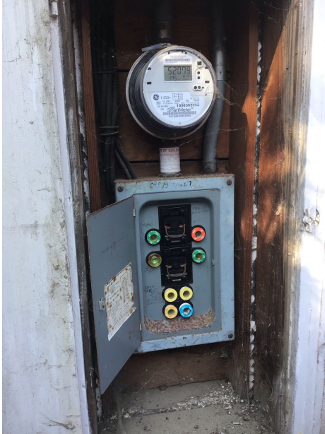
Today: 100-amp fuse box
