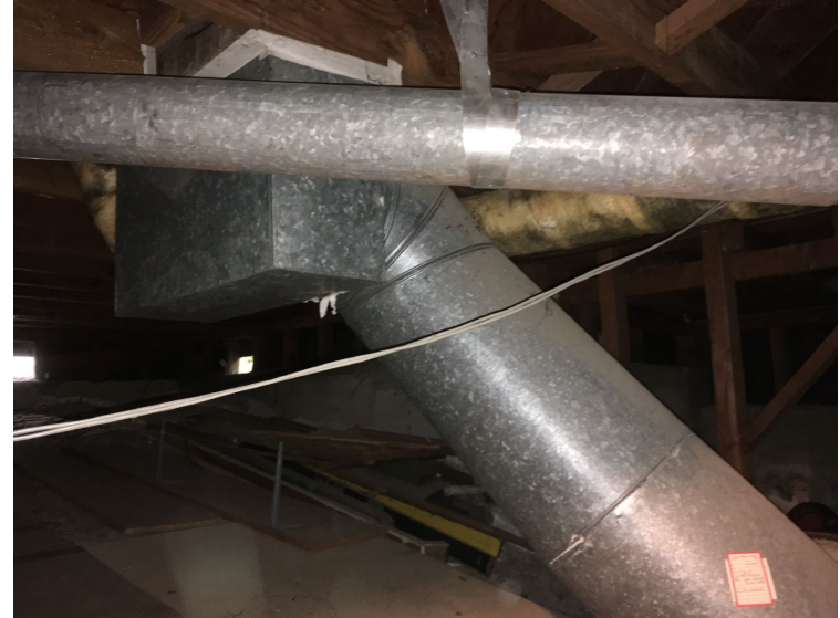
Today: Crawlspace, no insulation, limited duct insulation Optional: R-19 or R-30 for floors, insulate ducts
