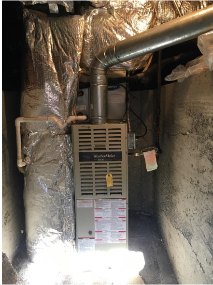
Today: Centrally ducted gas furnace
